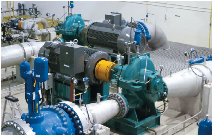
Airport Road Pumping Station
